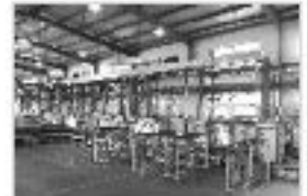
Automated Plating Line
